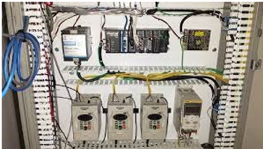
Fig 2. Typical mounting arrangement of AC drive units within control cabinet.
