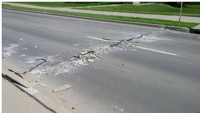
Figure 1.2: Destructive Effect of Thermal Expansion
